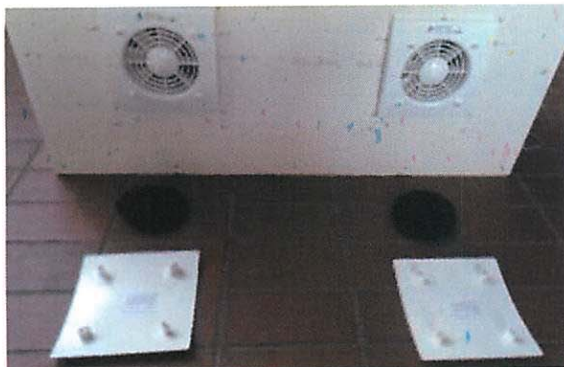
Bild 2: Indoor cover removed, filter
